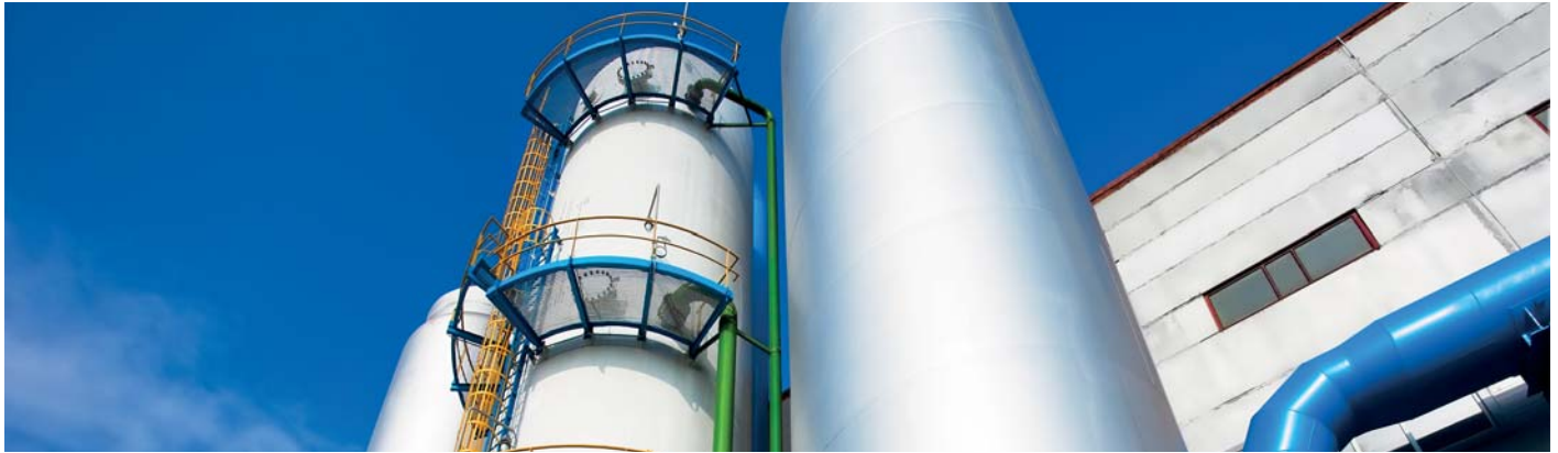
Air Separation Plant
